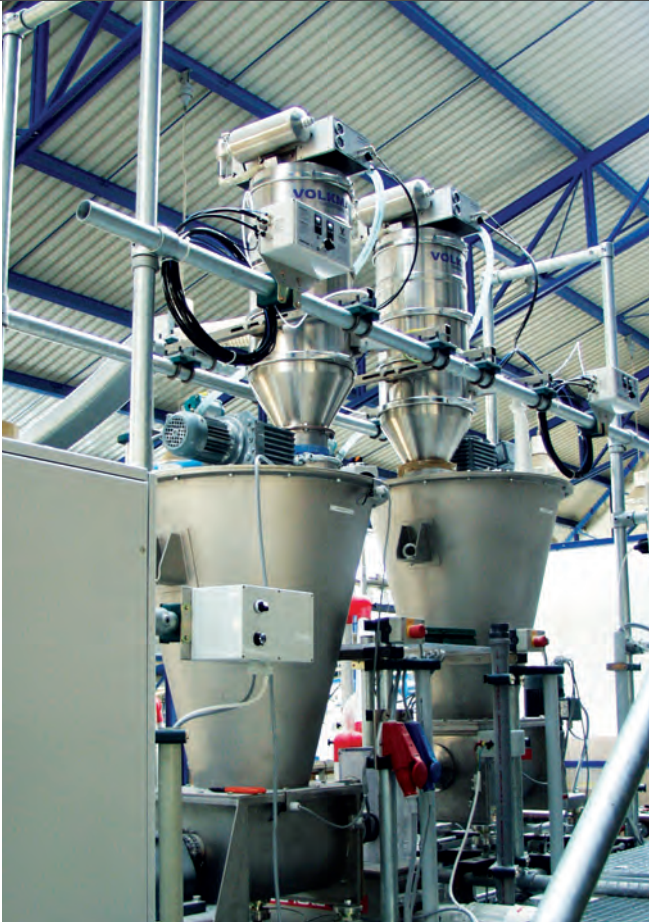
Two vacuum conveyors for loading loss-in-weight feeders.
